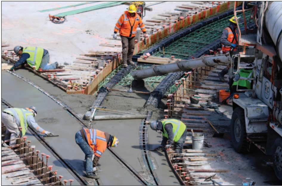
▲ Pouring and finishing concrete on the curve at Kilbourn Avenue and Milwaukee Street.
