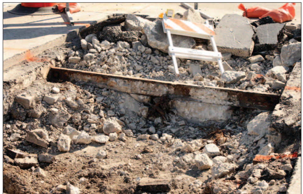
▲ Preliminary construction began in Spring 2016, starting with moving underground utilities where they were in the way. As is common in urban construction there were numerous things that had been buried or covered over. As seen here on April 23, 2017, the new streetcar construction ran into old TM rails. This rail on Plankinton Avenue had lain dormant since the end of the original streetcar service on Route 16 in June 1953.
